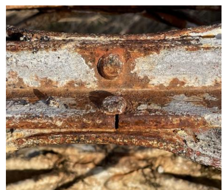
Sprung rivet can be seen on the left, and a fracture by the rivet on the right.
