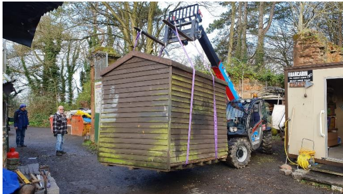
Members showing their expertise in moving a shed in preparation for wall repair
