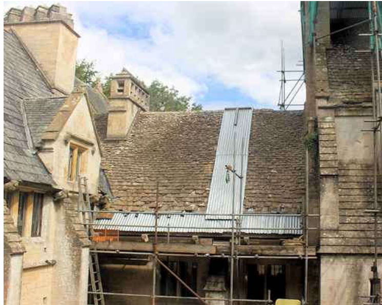
Ironing room roof before repair, showing corrugated iron patching, and to left, north range roof and chimneys awaiting restoration
