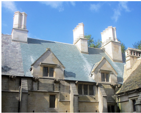
The new green slate roof on the N range, with restored chimney stacks, and to the right, the new Cotswold slate roof on the ironing room
