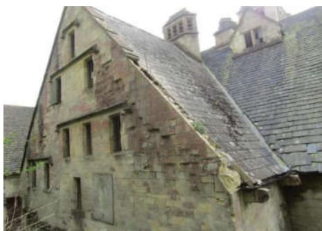
Left: the damaged brewery gable
