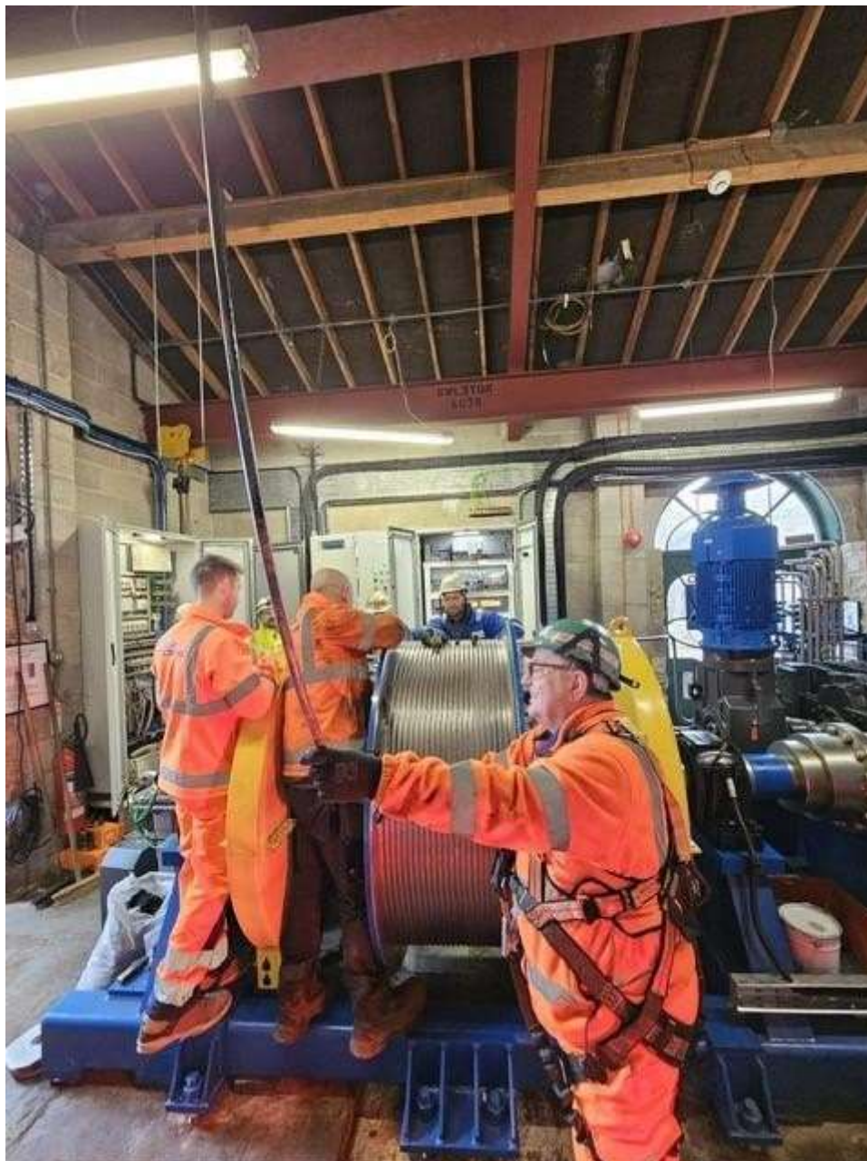
Installation of new winding engine that operates the cage to go underground
