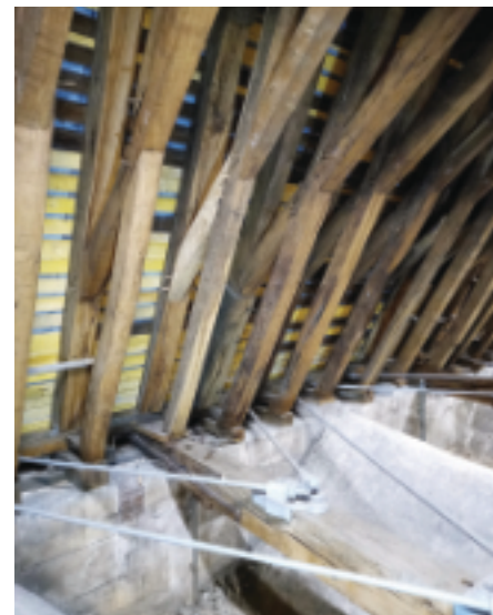
Nave roof transition above porches indicated by the brick infill of a timber beam slot
