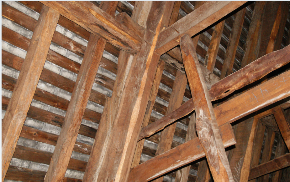
Fig 10 Medieval timber reused as rafters and the 18th century truss supporting the roof
