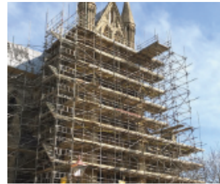
The lesser transept south roof was the first restoration project to be completed in May 2021.
