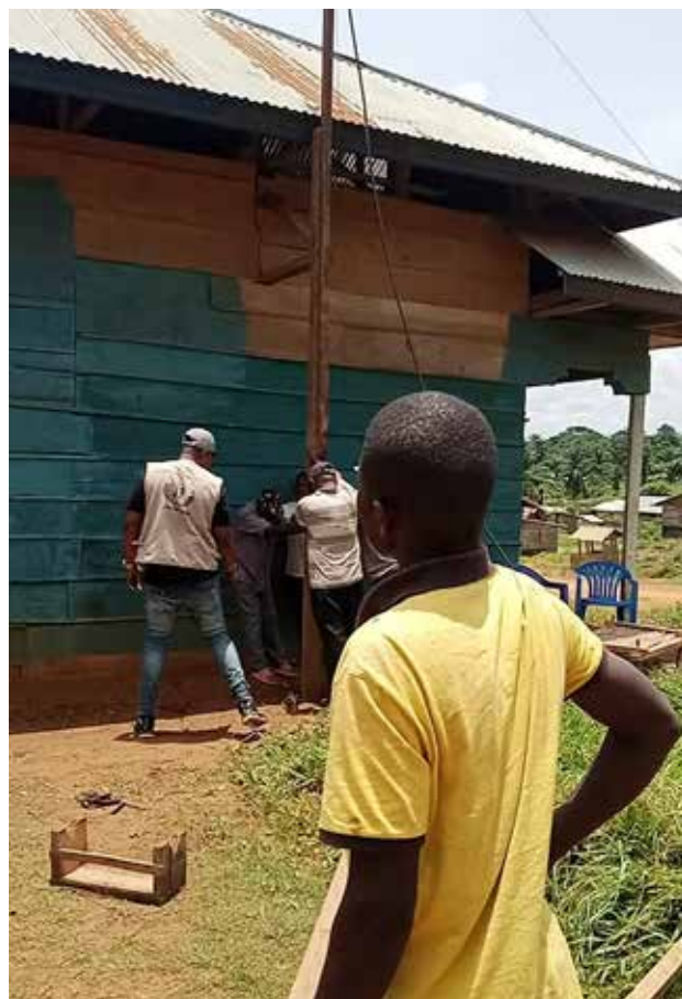
An antenna is installed for the Mayuano Community Radio in Ituri province in DRC as part of our project, 'Madini kwa Amani na Maendeleo', in partnership with Justice Plus. This was an action point in the community's local security plan, to improve access to information and social cohesion in this artisanal gold mining area. Photo: © Justice Plus
