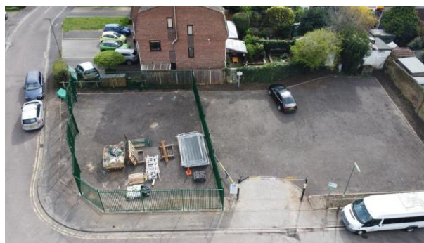
Aerial view showing the high security fencing as installed around the new compound, end of March 2024
