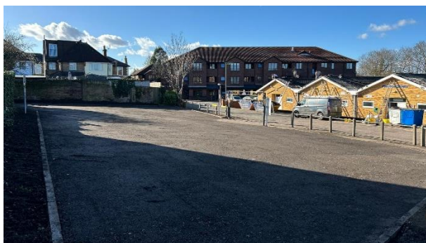
Ajax and Warspite volunteers combined efforts to complete site preparation works in February 2024
