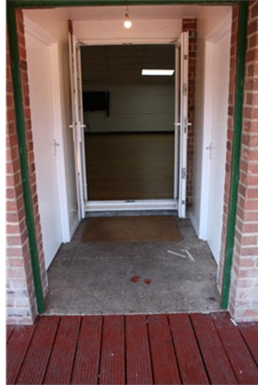
Doors from balcony do not allow level access into the Main Hall
