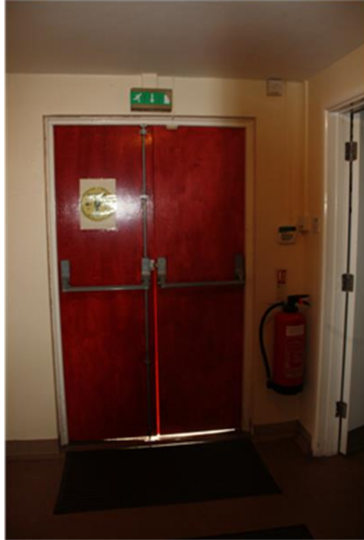
Front door – not very secure and no cover to prevent rain damage
