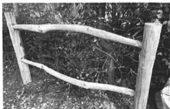
A section of the fence built in Smallheath Eco Park for the peace garden by youth from Birmingham.
