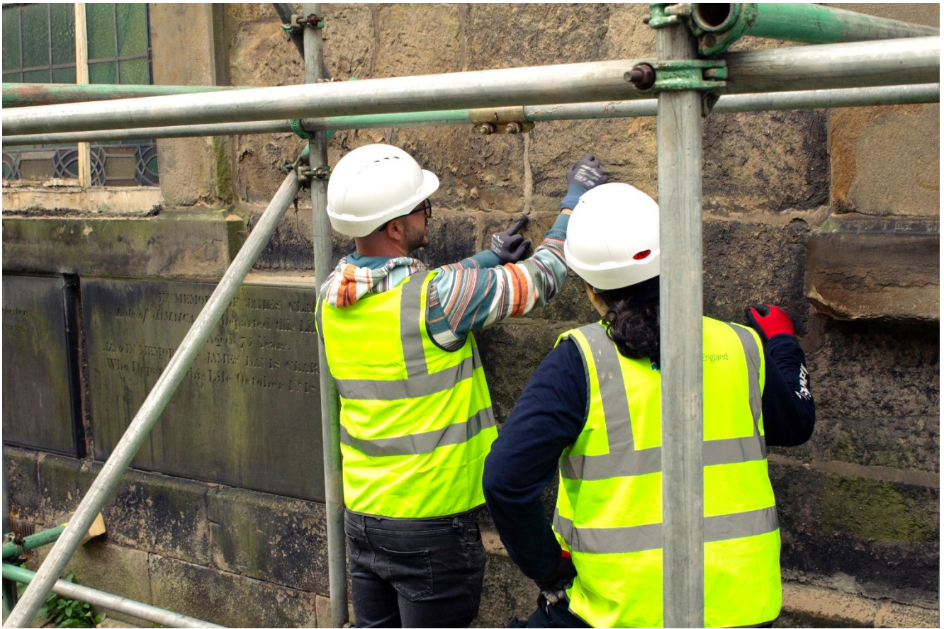
Apprentices at the summer school inspecting old lime mortar on the exterior of St John's Church, Lancaster (CCT).
