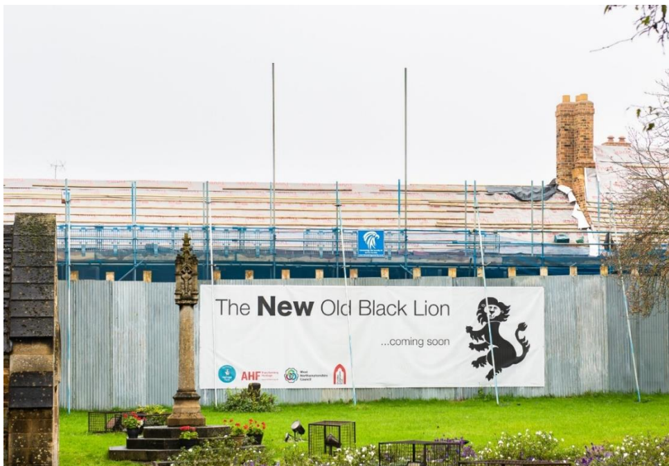
A view of the scaffolding on the Old Black Lion pub, viewed from the churchyard of St Peter's Church (Stu Vincent Photography)
