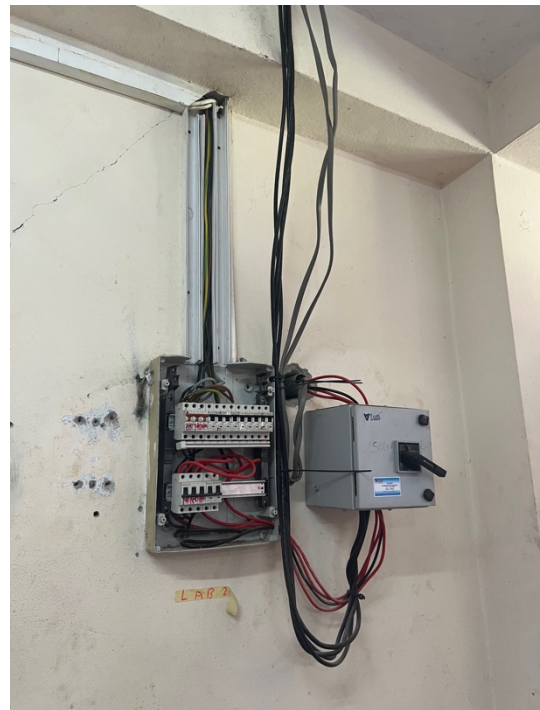
Unsafe fuse box with wires
