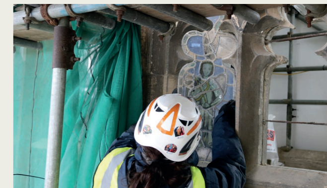
Repair of the masonry and glazing along the south wall Photo: Winchester Cathedral
