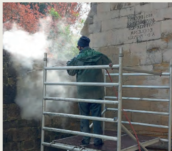
Curle's Passage cleaning, conservation, and some replacement of decayed stonework 2024 Photo: Winchester Cathedral
