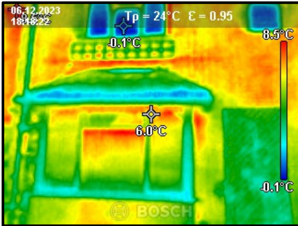
A Thermal Image of a Waverley Property
