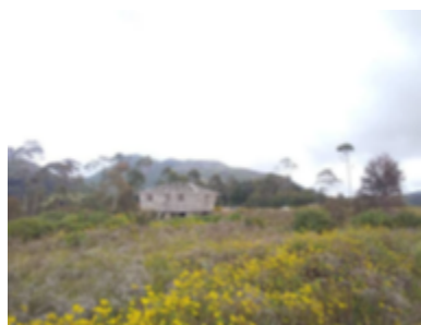
The research centre on Mount Mulanje before the roof is put on.
