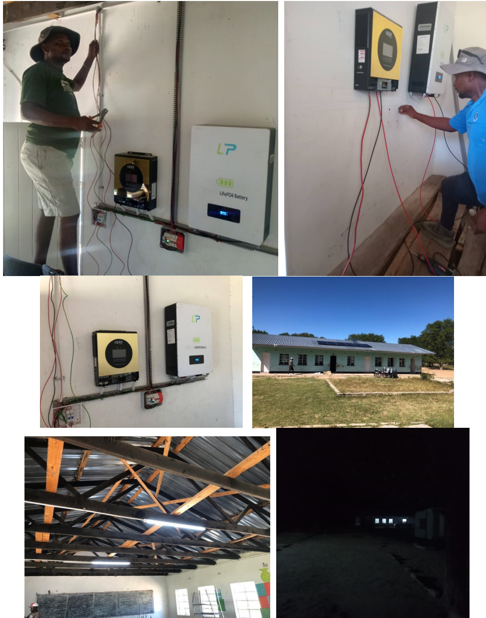
Power installed at Mlevu Primary School
