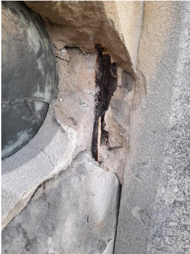
Figure 2 Damaged stonework requiring urgent attention.
