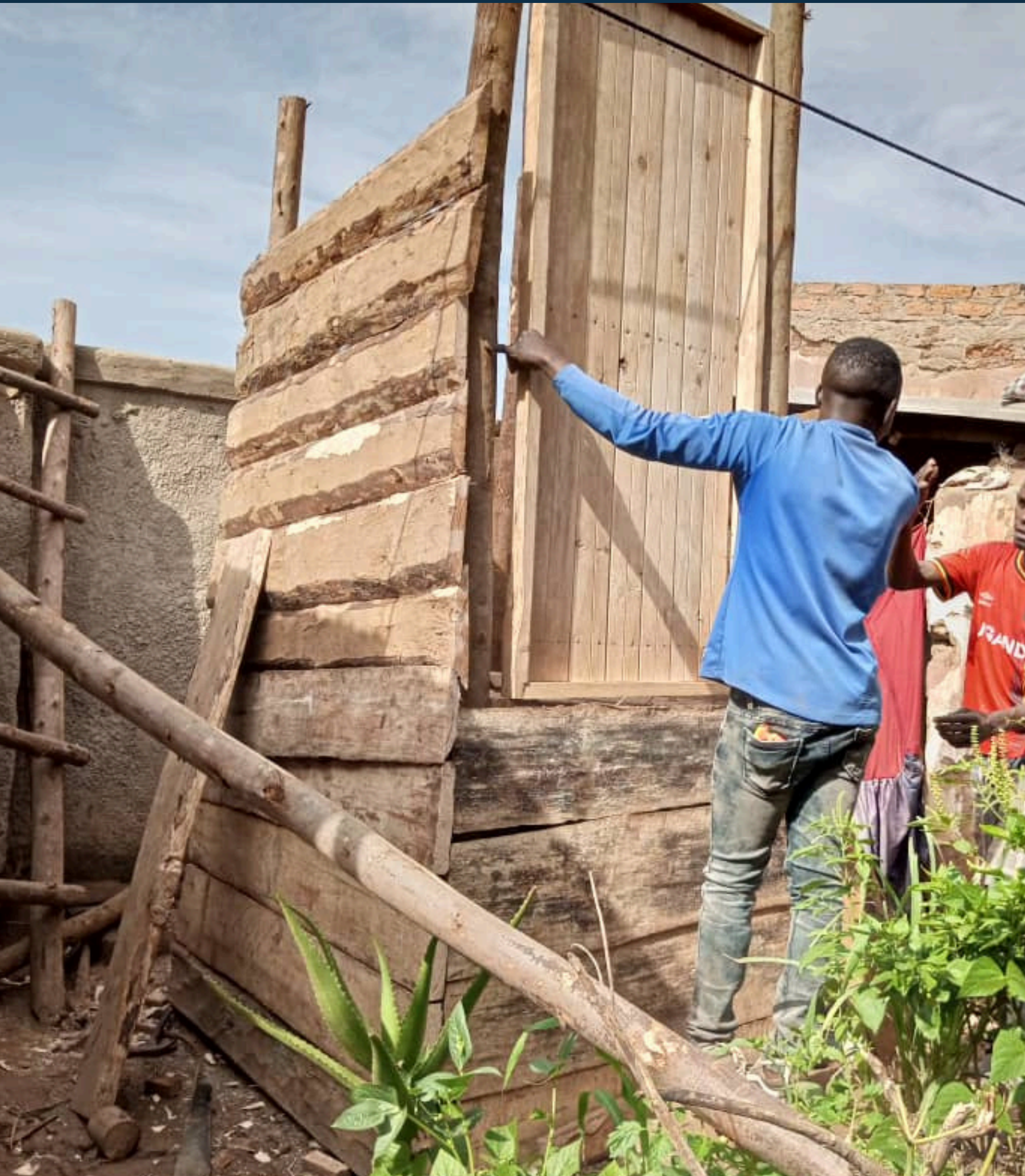
Construction of Ecosan Toilets in Nakivale Uganda by partners YICE as part of our Regenerative Camps settlements project
