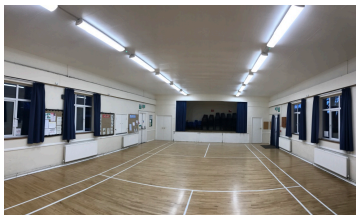
Main hall general lighting
