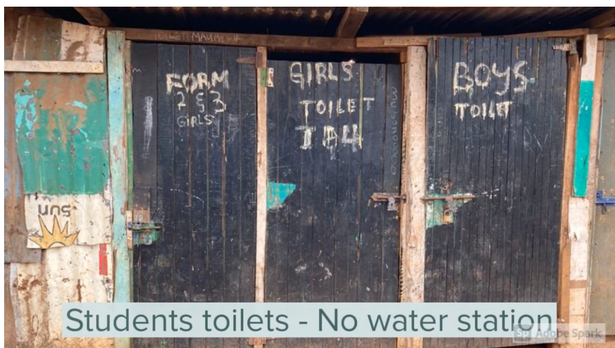
Student toilets at Silver Springs High School before renovation work began.
