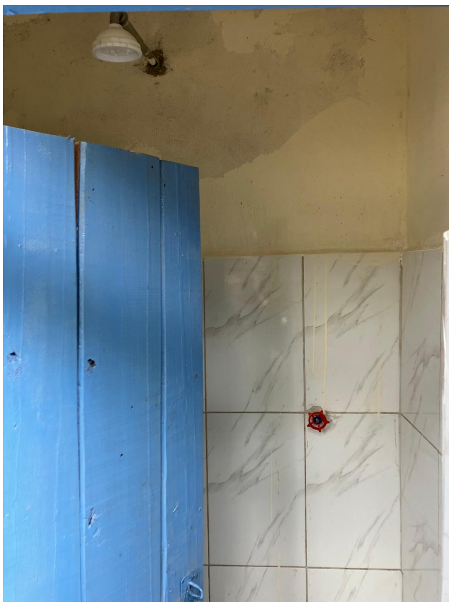
Changing and shower cubicle within the new toilet block at Silver Springs School.
