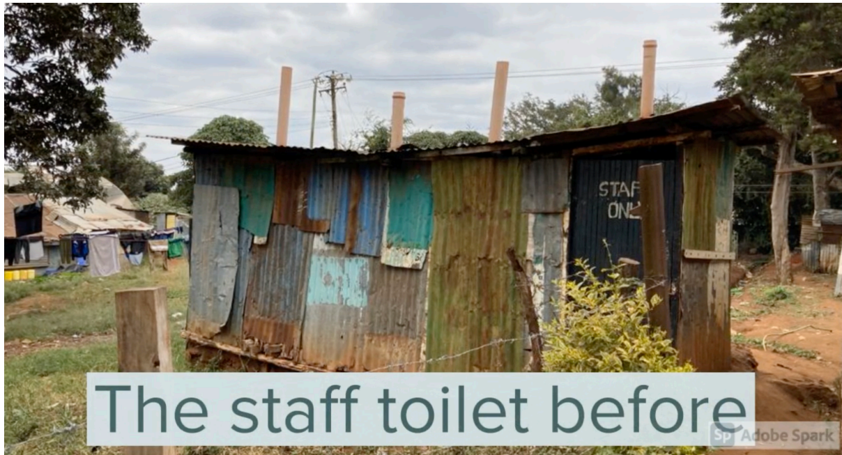
Staff and student toilets at Silver Springs High School before renovation work began.
