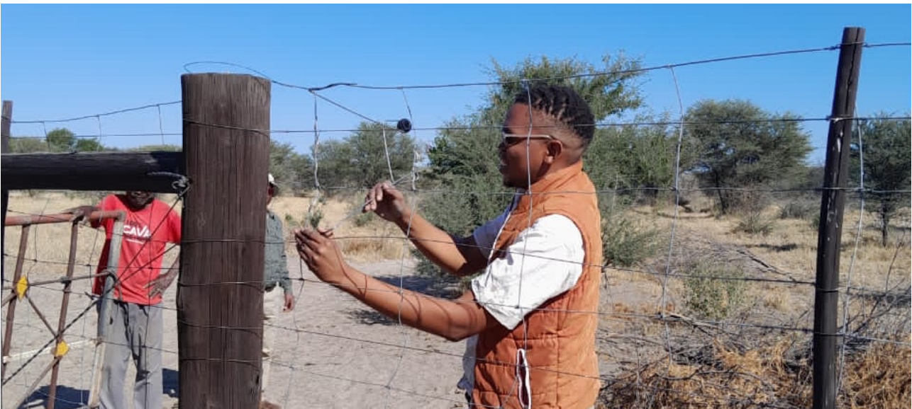
Photo 9: Efa Community Outreach and Education Coordinator, Mr Walona Sehularo, demonstrates connecting offset brackets to an electric fence.
