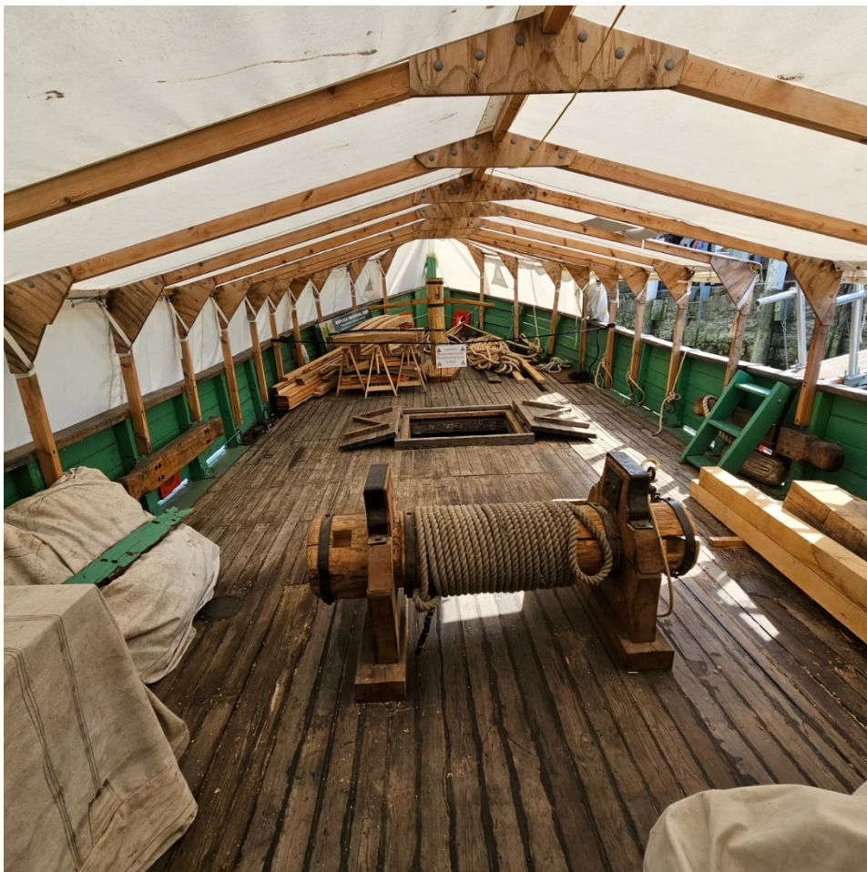
Windlass and Capstan Installed
