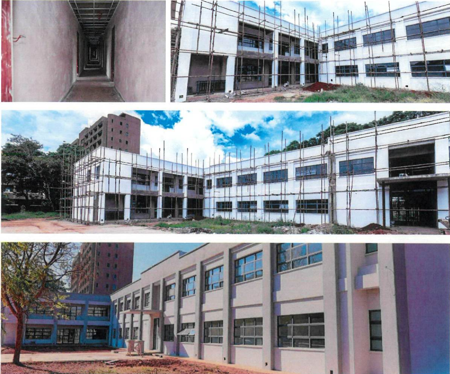
Final stages of the construction of the National Emergency Operations Centre in Harare, Zimbabwe
