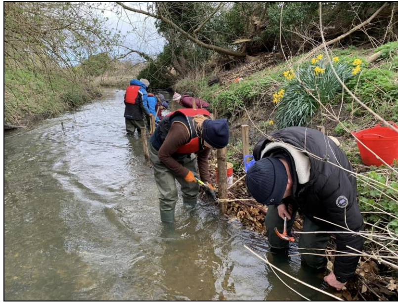
Installing brushwood bundles on the Lark near the Lark Valley Golf Course in April
