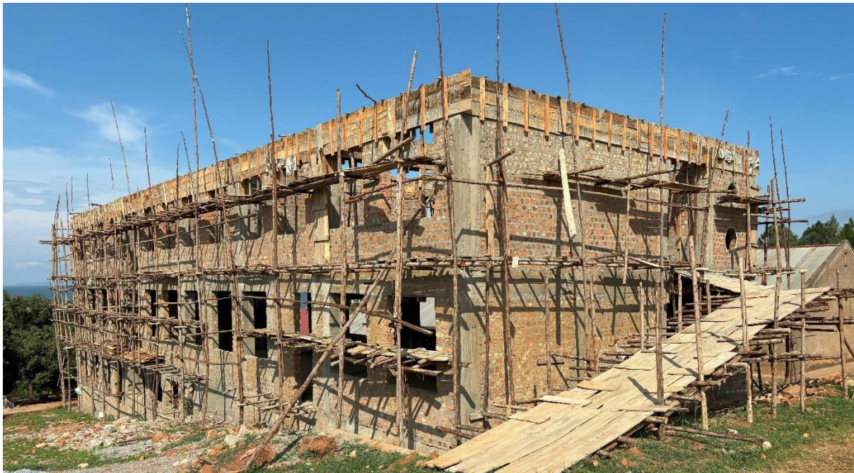
FIGURE 4. CLASSROOM CONSTRUCTION MAKING GOOD PROGRESS. PHOTO FROM MONITORING TRIP BY DANNY MORRIS (CEO) SEPTEMBER 2024.
