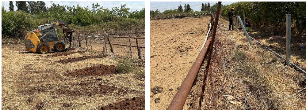
Above: Building work begins – the unstable old fence is the rust coloured one, the new one is behind it. Below: The donkeys in their now safe enclosure with the new fence.
