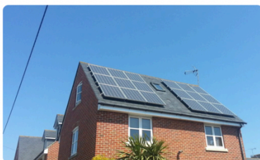
Solar PV Systems & Biomass Heating
