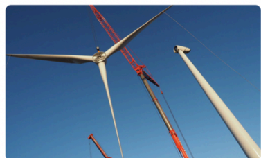
Wind Turbine at Alvington Court
