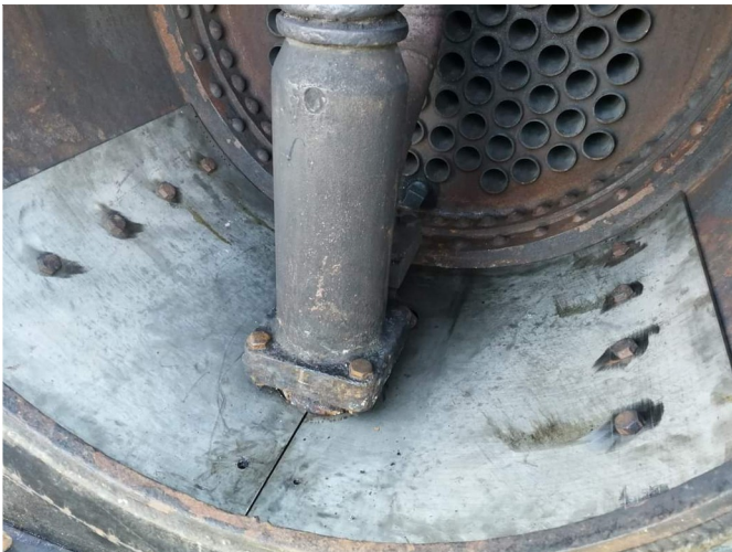
Gelert's new smokebox floor (left) and baffle plate (right) being made and fitted by our trustees and volunteers. (photos: Myles Jones)
