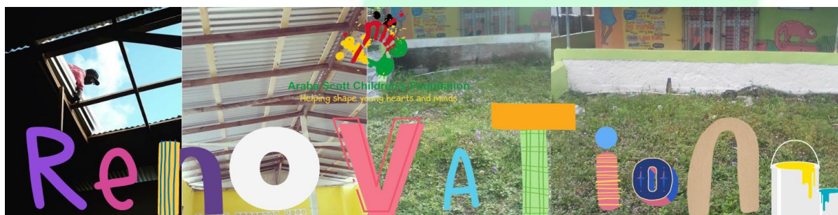
Figure 4 A photo of Prophet (our builder) working on our new roof, the completed roof, and the before and after photos from painting the veranda wall outside Barnes Hall
