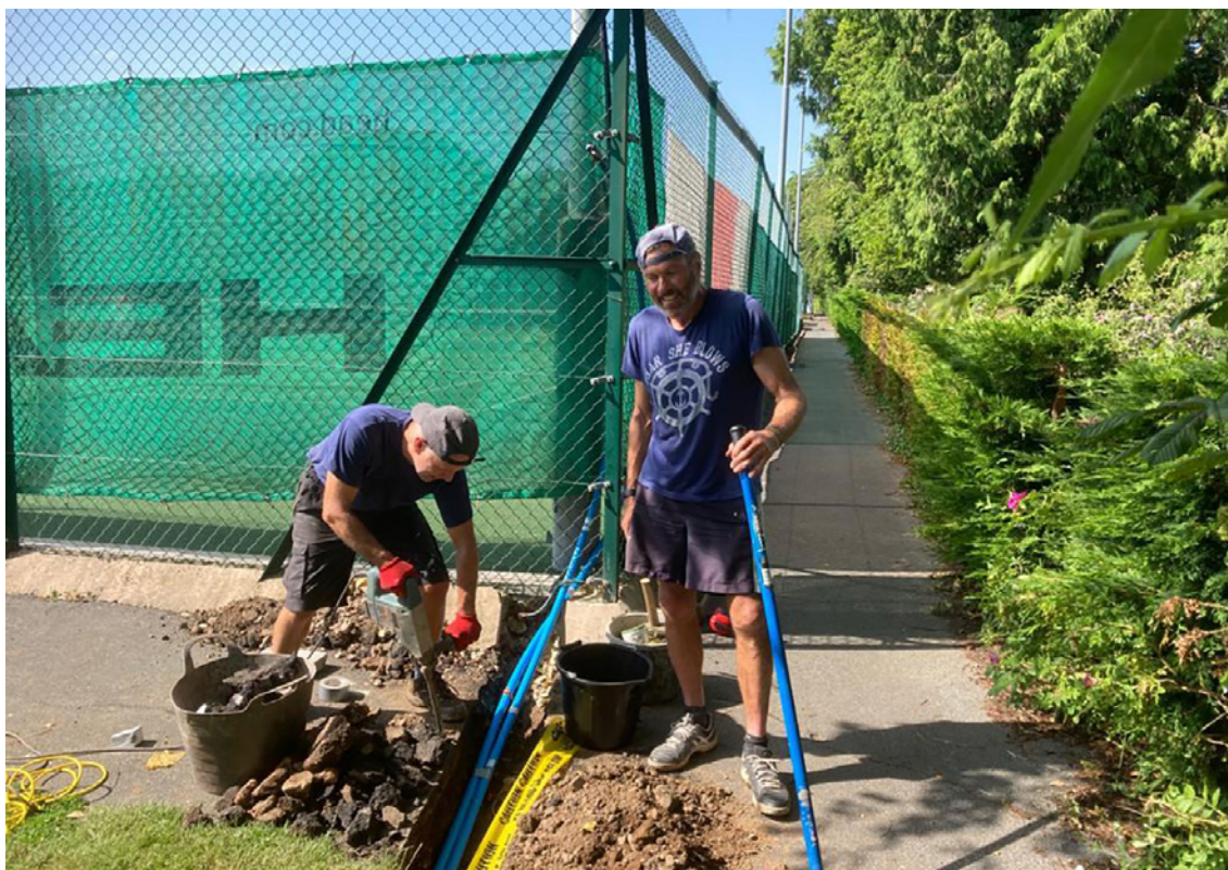
Paul Thomas and John Callaway digging a trench for the court 4 LED lights wiring
