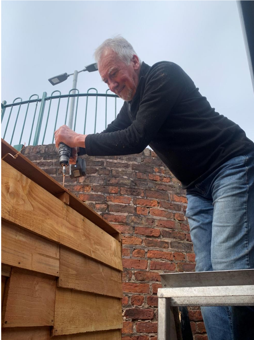
Volunteer (and Trustee) Peter Graham at work on the erection of a storage shed to the side of the Centre – April 2024.
