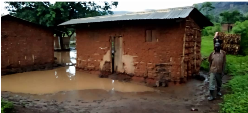
3 images – aftermath of flooding in April 2024
