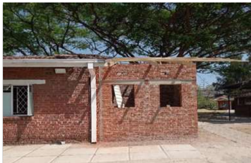
Care Unit toilet which is being extended so that it improves the sanitary facilities for admitted patients.
