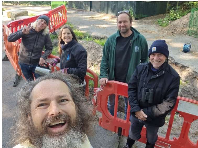
Fig 3 – Start of pond build in Woodland Walk (Credit photo from Cllr Farqhar)
