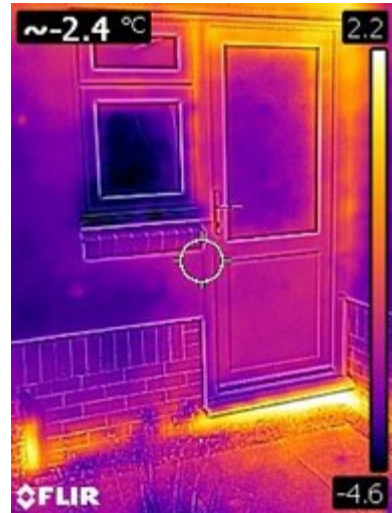
Infra red image showing heat leakage
