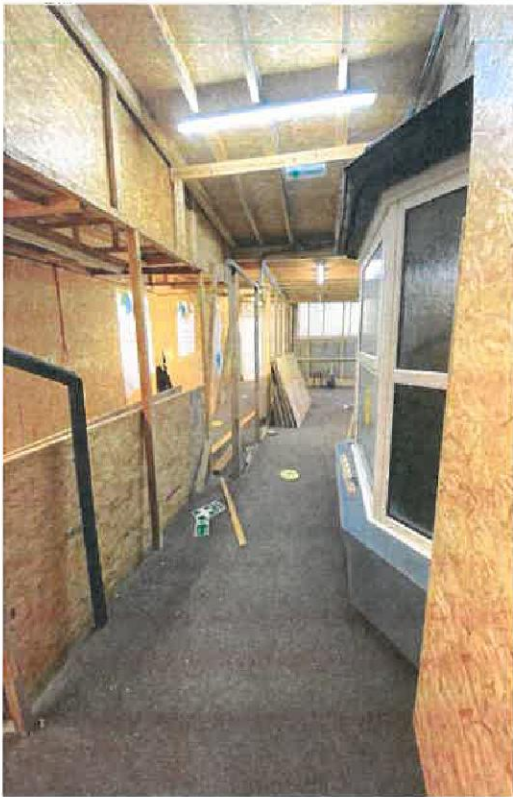
Removal of temporary wooden structure linking main hall to the front entrance
