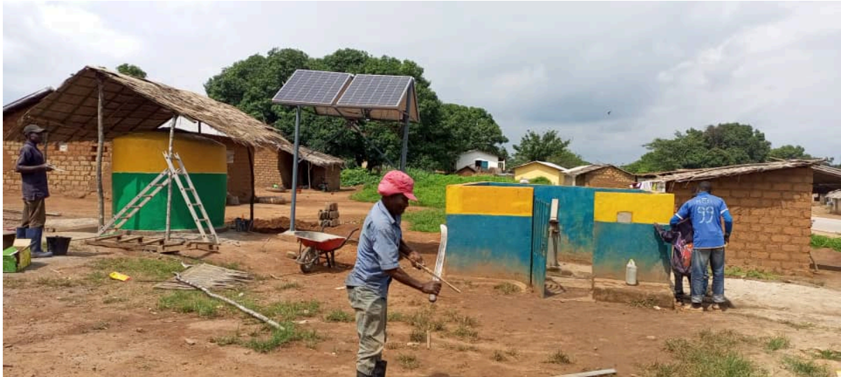
Solar pump retrofit of Cameroon Catalyst well in Mbangue
