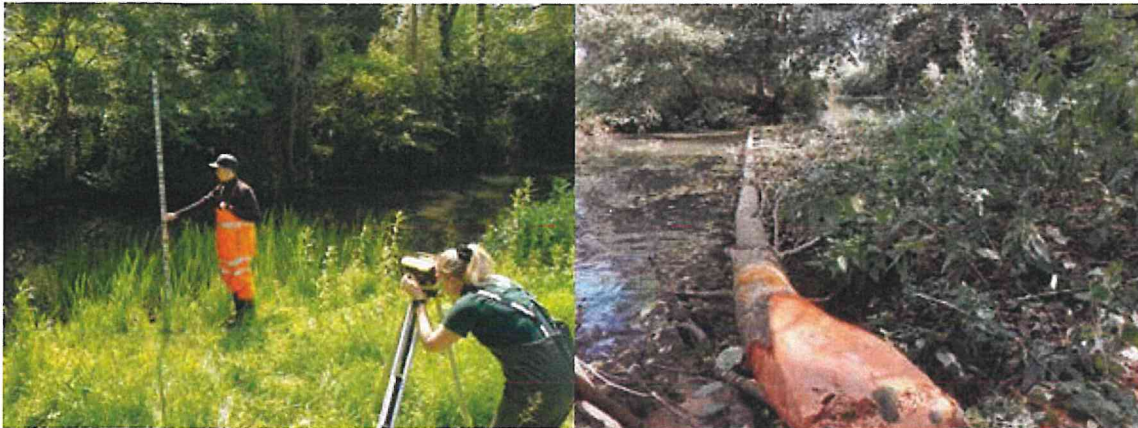
Image: the BART team undertaking a detailed site survey, and on the right, a hinged tree installed on the Sherston Avon, to improve flow diversity and habitat to support wildlife
