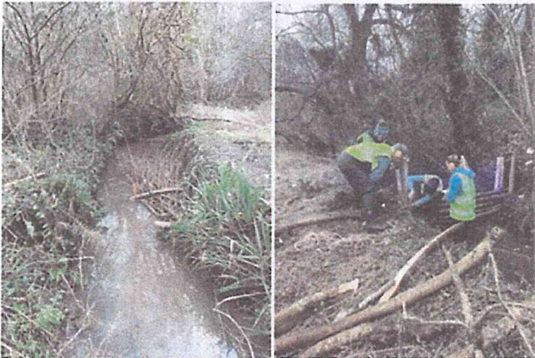
Image: After installation of berm along the right-hand bank; construction of a "leaky dam" with support from volunteers.
