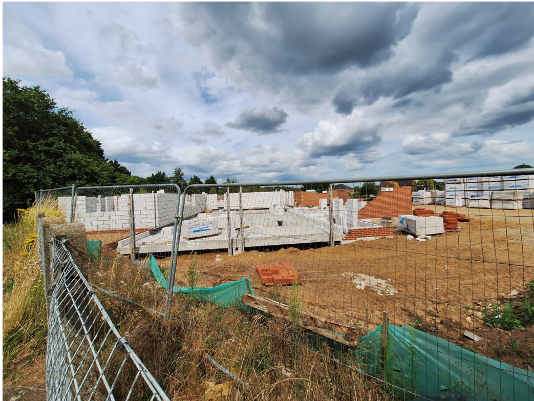
Construction of the hall begins. The base is in place in July 2025.
