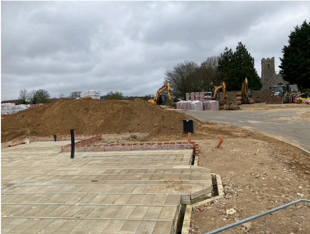
View of site in on 31 March 2024. Hall location is where the digger are. The line of the road and the base of one house
