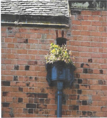
8. Blocked hopper head
