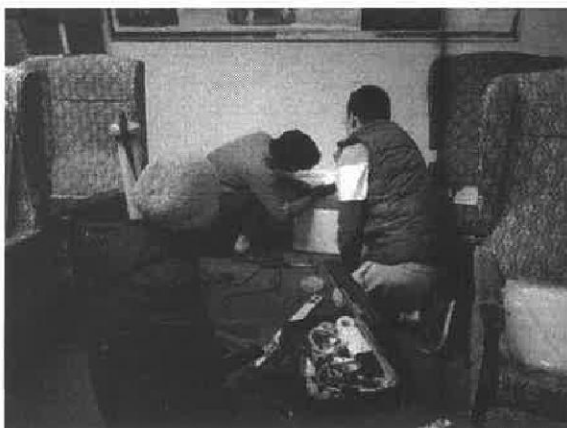
Volunteers donated some heaters and helped to install them for the Centre in Dec. 2021
