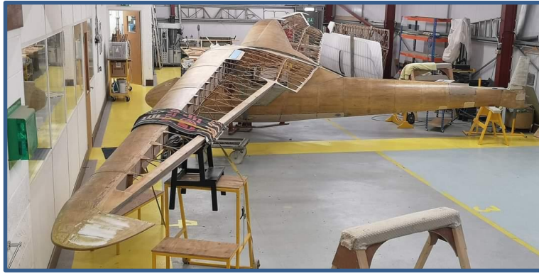
Work underway on the Spalinger S21h showing the intricate wooden structure of the wings, much of which needed to be repaired.
