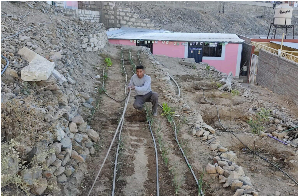
Drip-irrigation school vegetable garden
