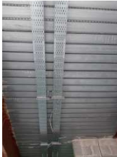
This image shows the channel trays that were fitted on the first floor.
