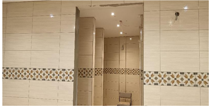
The image above shows the first floor wudu khana & toilet walls tiled and spot lights fitted.
