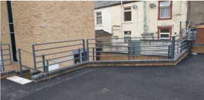
The image above shows the safety railing installed on the retaining wall.
