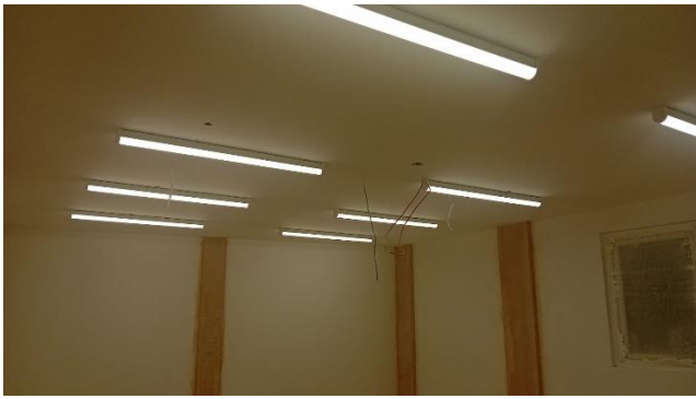
The image above shows the lights fitted in a classroom.
