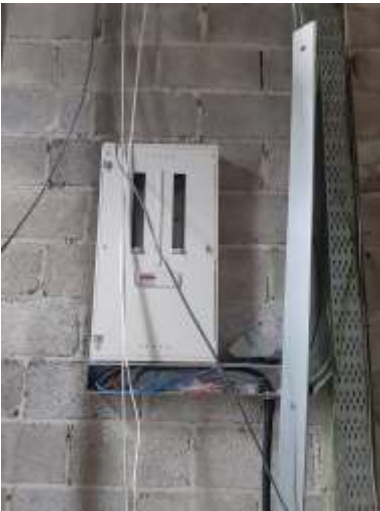
This image shows the meter distribution board on the first floor.
