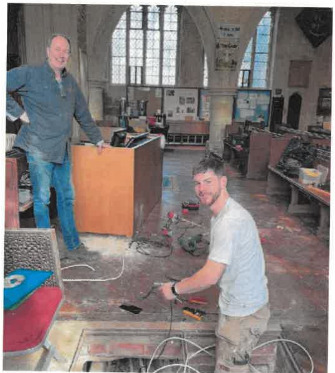
Installing the new sound desk in March '25
