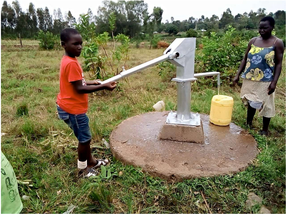
One of the many hand pumps repaired. This was a new replacement pump.
