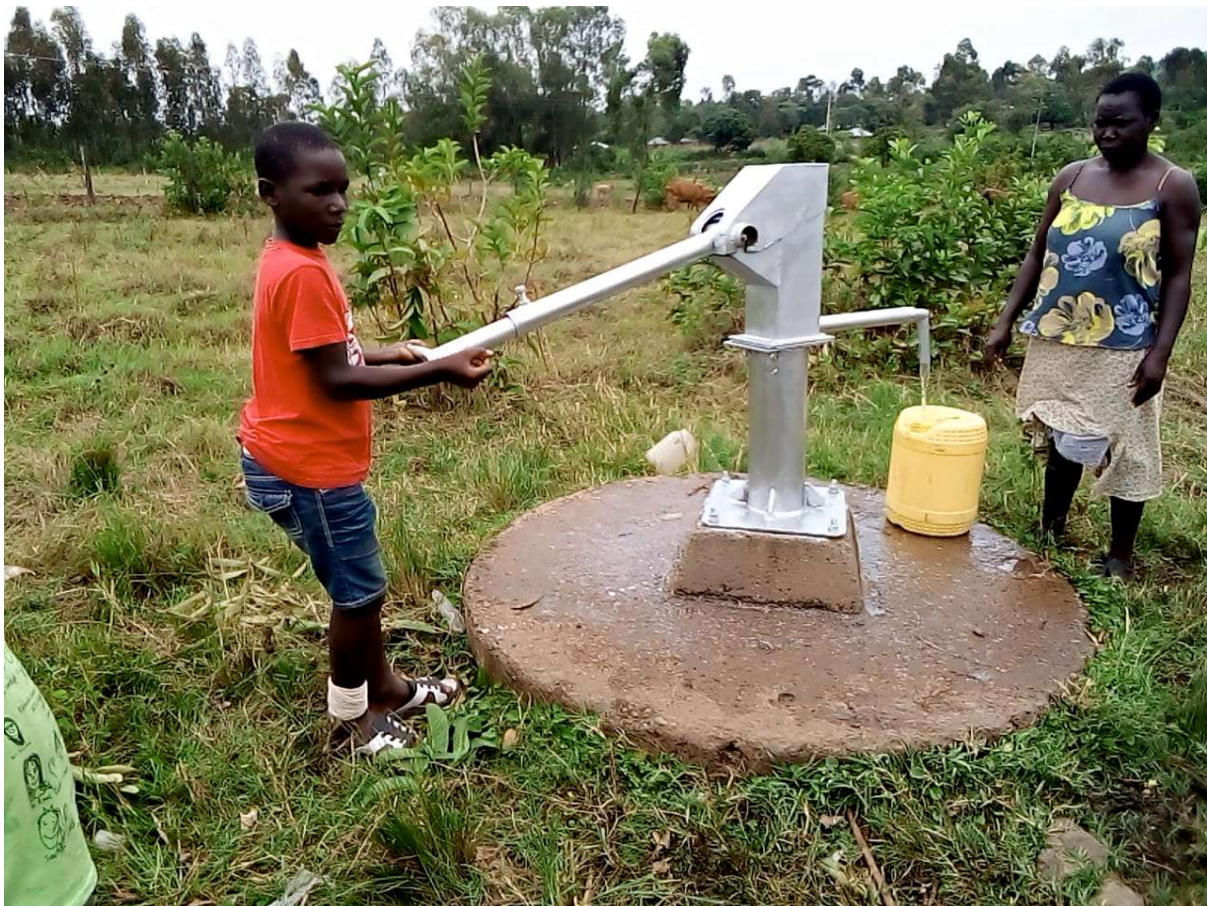
One of the many hand pumps repaired this year. This was a new replacement pump.
