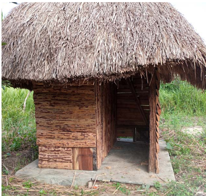
We are also building composting toilet blocks at the Peace Centre in order to showcase its many benefits to the wider community.
