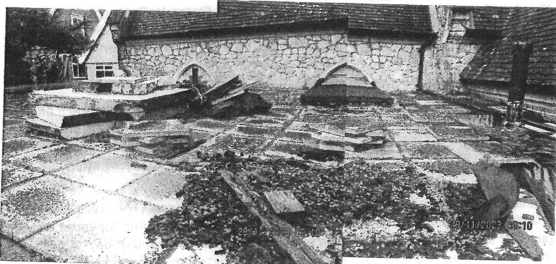
The vestry roof after partial removal of slabs and cladding, looking for water ingress.
