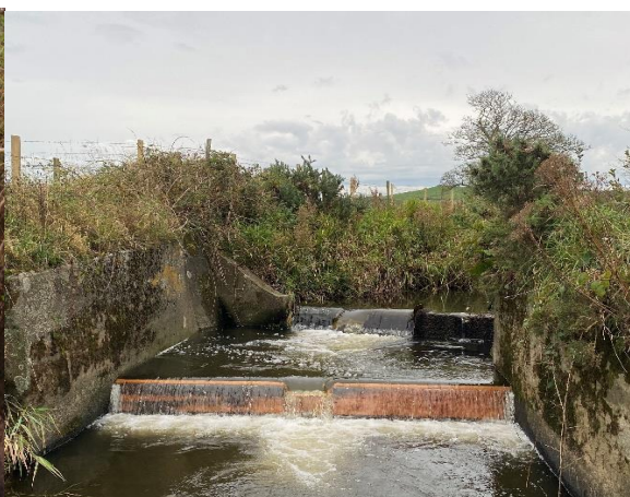
Weir with notch and removable timber pre-barrage
