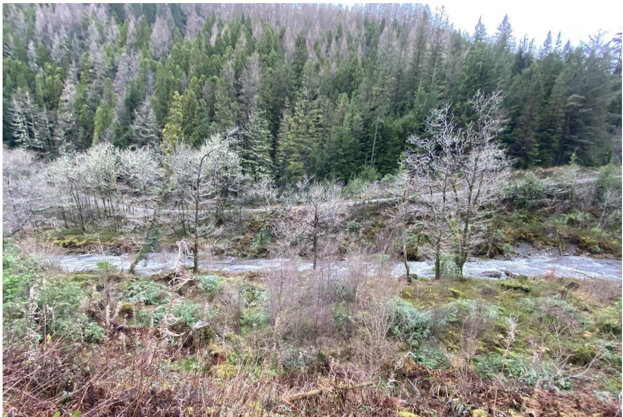
The cleared corridor between the two forestry roads showing brush piles in the foreground
