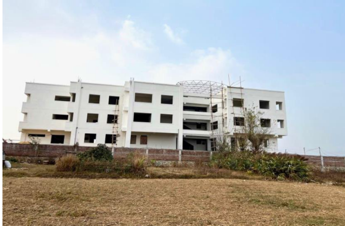
Siddhasthali Rural Community Hospital
