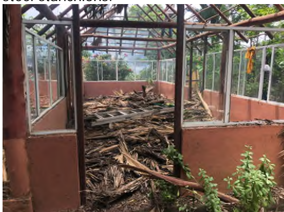
2 Refurbishment following the 'Ranch' roof collapse
